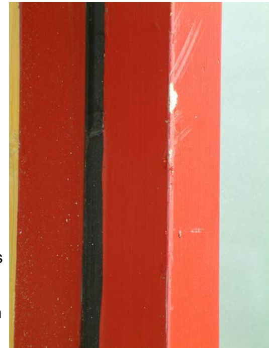
Plate 4 Attempted repainting of an aluminium shopfront
