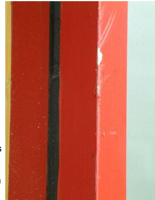
Plate 4 Attempted repainting of an aluminium shopfront
