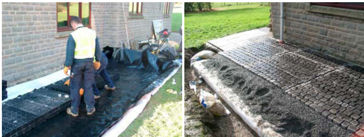
Installation of a rainwater harvester system below a permeable concrete block surface
