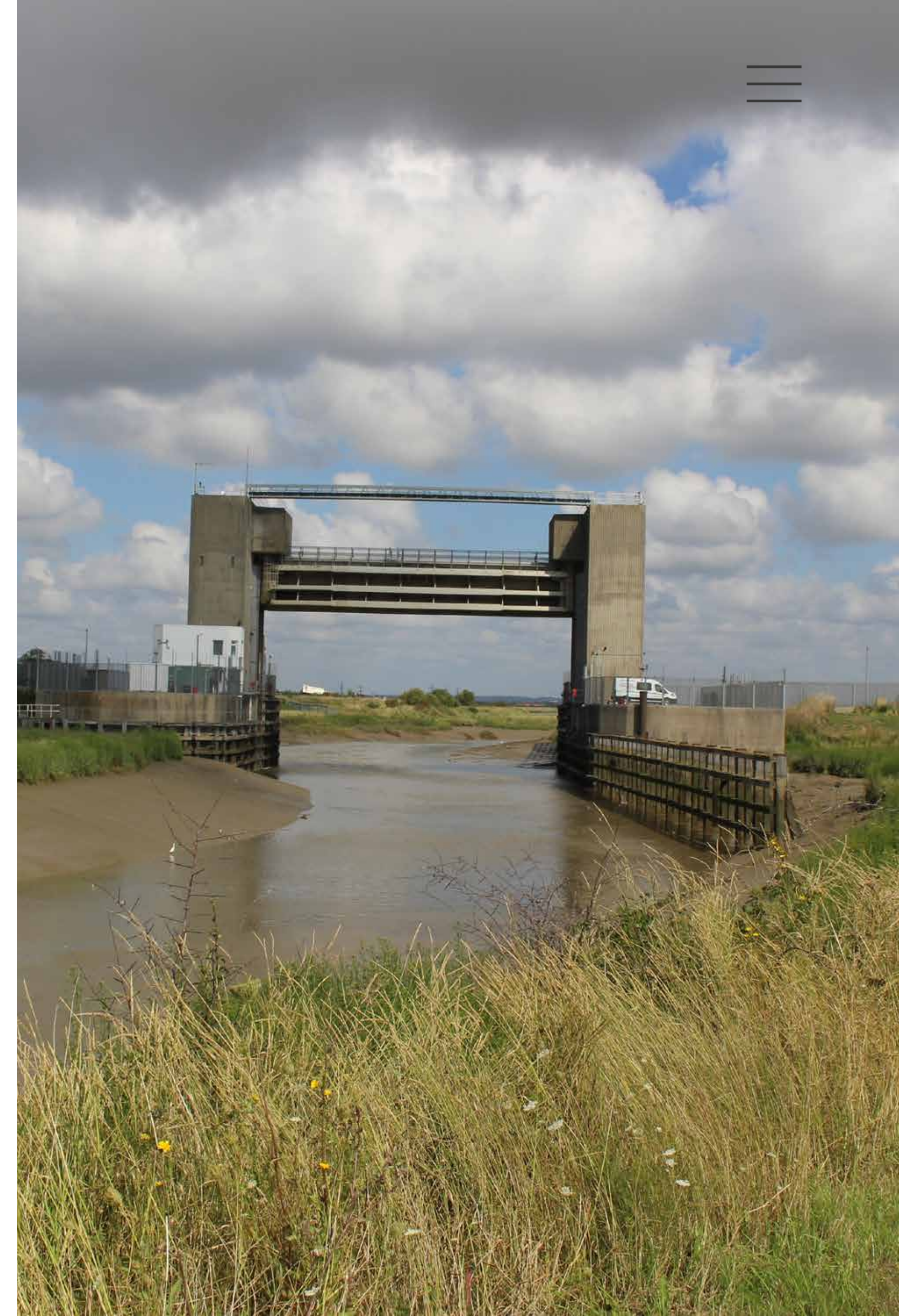
Figure 119. Dartford Creek Barrier
